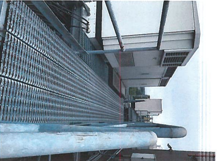
Equipment Platform Cabinets (Typ.)
